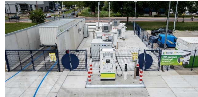
Hydrogen Re-Fuelling Station, 2021
